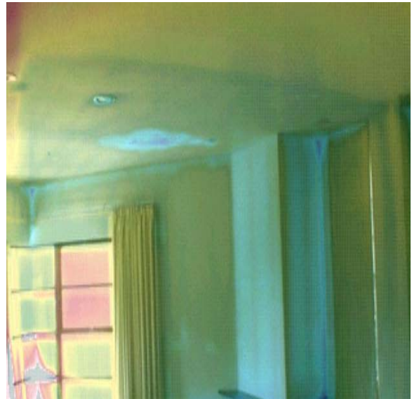
Infrared Thermal Image under deck
