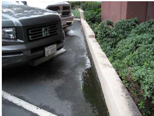
West elevation water seepage
