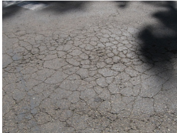
Typical alligatoring at parking
