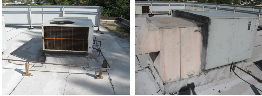
Roof mounted Trane mechanical units.
