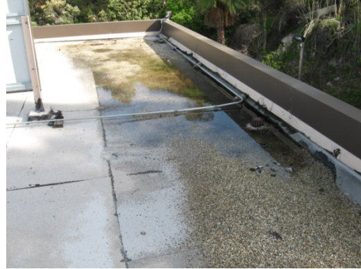
Ponding at Built-Up Roof
