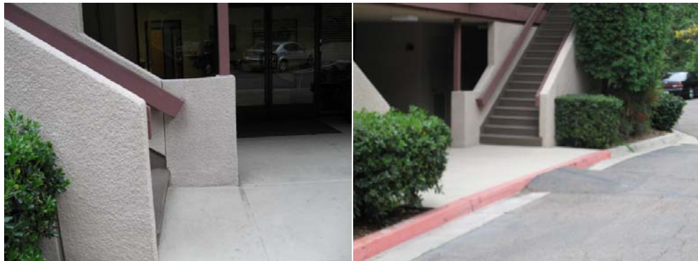
Handrail does not extend 12-inches beyond landing Access ramp may not be ADA compliant
